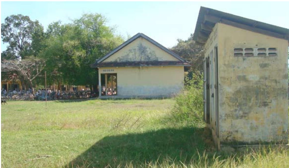
A school and its pour-flush latrine surveyed by CDRI researchers for the 'Knowledge, Attitude and Practice on Sanitation and Hygiene' project, Kompong Speu province, November 2011
