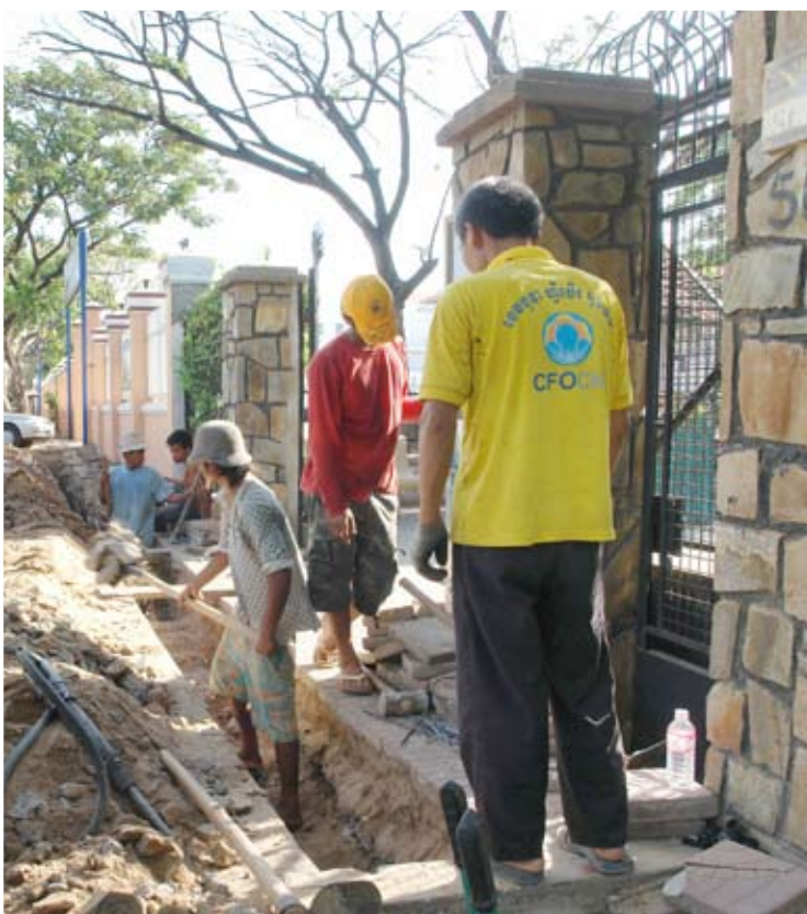
Cambodians benefit from low priced Chinese imports and the jobs and infrastructure created through Chinese investment projects like the optic cables being laid in Phnom Penh, March 2012
