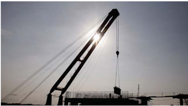
Construction of a new container terminal at Phnom Penh Autonomous Port, which is set to profit from the expected bigger flow of goods with the start of the ASEAN Economic Community, Kien Svay district, Kandal province, August 2013
